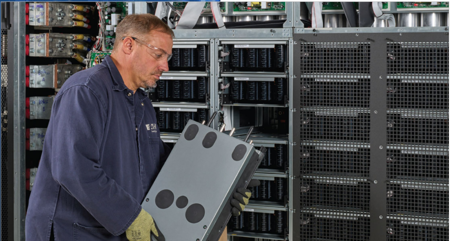
Eaton technician inspecting an Eaton 9395XC UPS.
